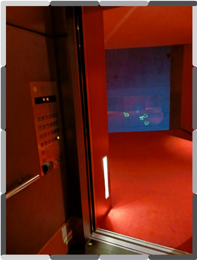
Looking out from the cab into a red hallway on the eighth floor
