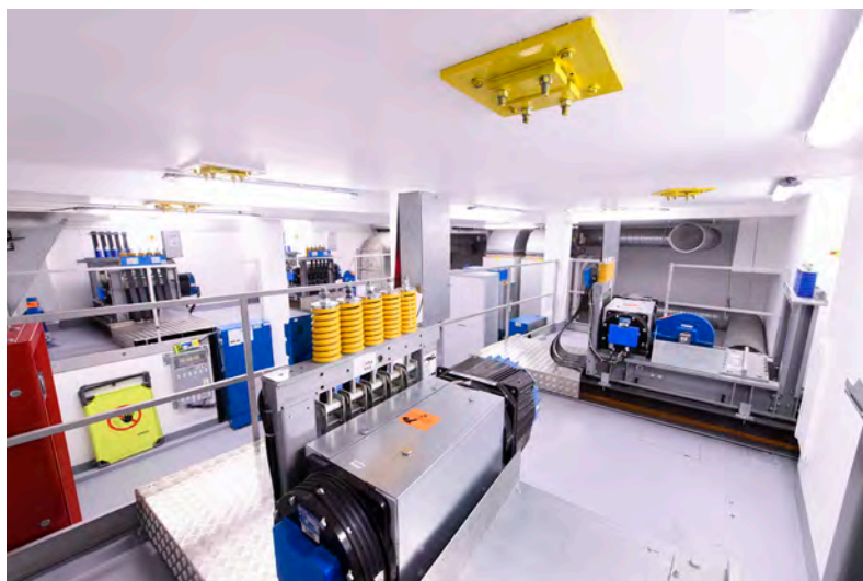
Lower bank machine room after
