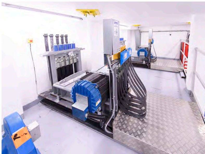
Lower bank machine room after
